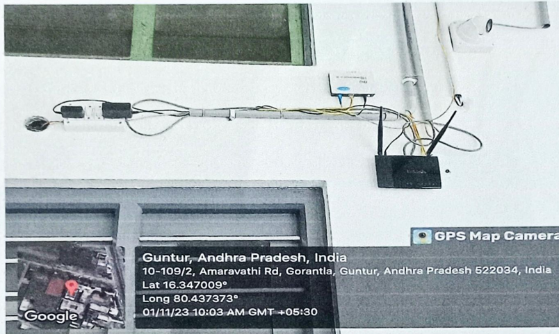
Wi-Fi router at Skill development Lab
