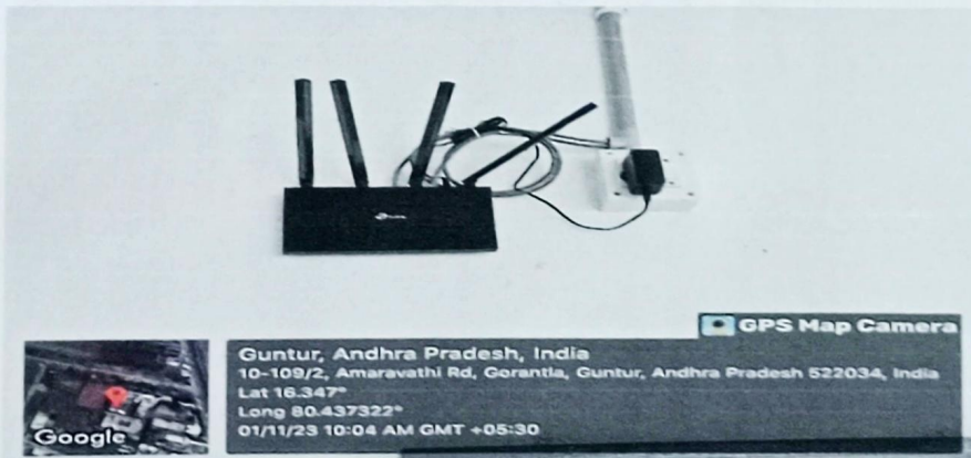
Wi-Fi router at Corridor
