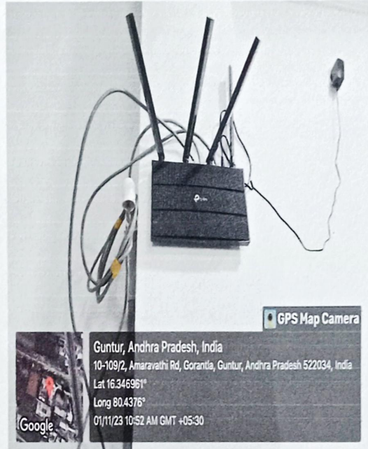
Wi-Fi router at PG Computer Lab
