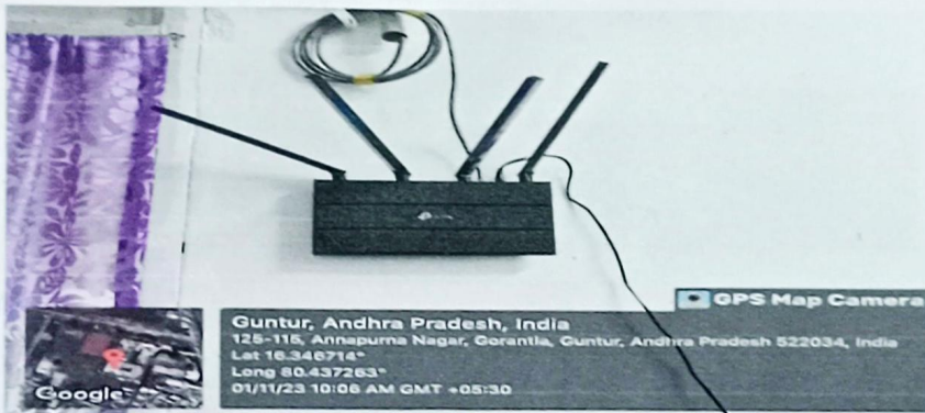
Wi-Fi router at UG Computer Lab
