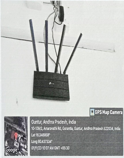
Wi-Fi router at Corridor
